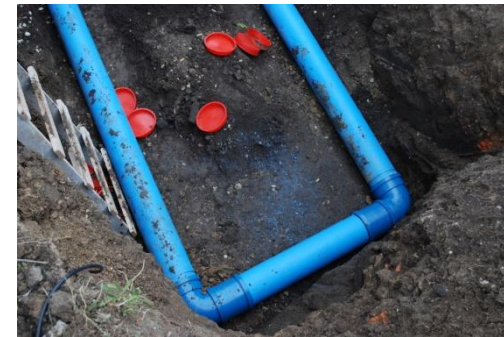
Pipe of the EAHX
